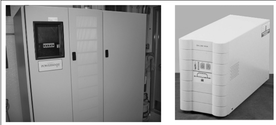
Figure 7-2 Redundant three-phase UPS system for data-center equipment and front and back views of a small UPS box, adequate for one rack or a few servers.
