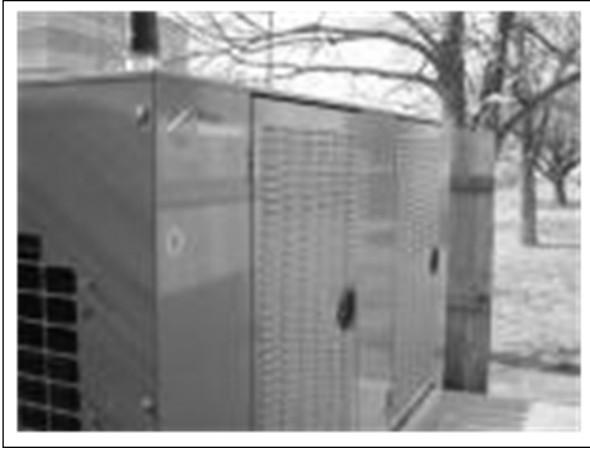
Figure 7-3 Redundant generators located outside a data center.
