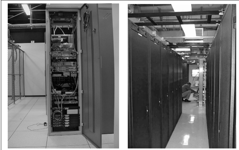
Figure 4-1 Data center with locked cabinets and cables but with no raised floor.
