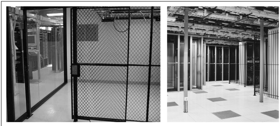
Figure 4-2 Data center with no raised floor. Cabinets and stand-alone equipment are in cages.
