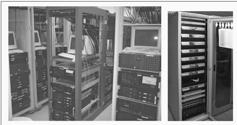
Figure 3-1 Cabinets and racks in a data center.
